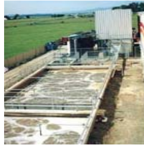
Modular treatment Systems
